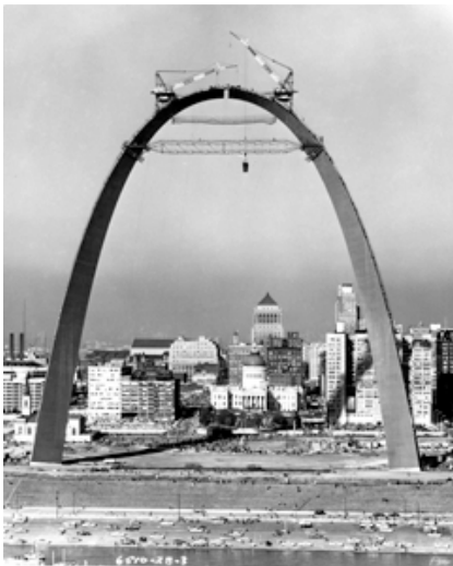
Eero Saarinen United States Jefferson National Expansion Memorial, St. Louis, Missouri, under construction, 1965 From the Collections of Arteaga Photos Ltd.
